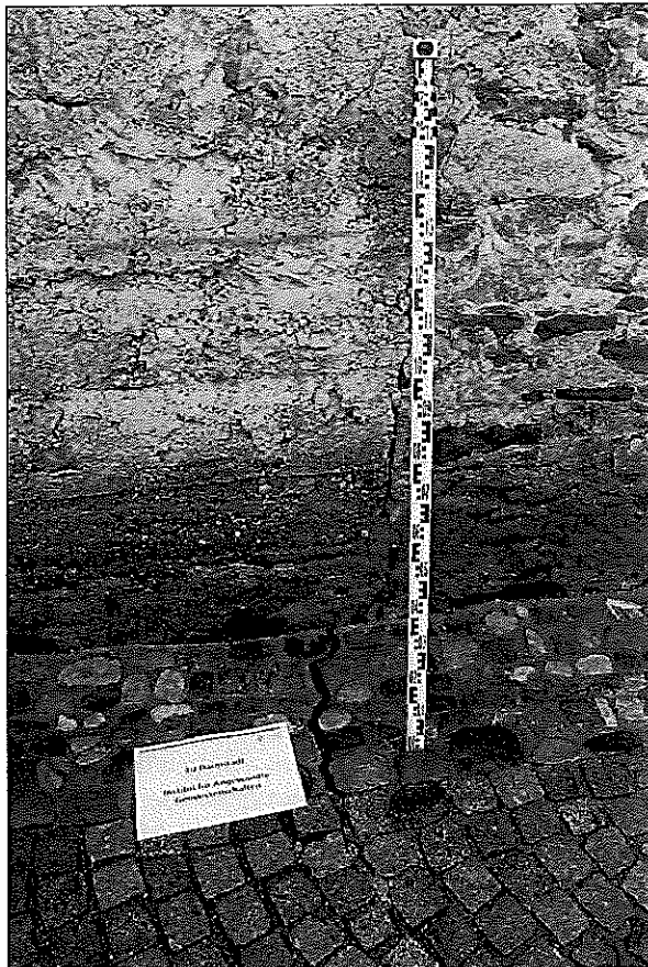
Fig. 4: Crack in the street "Jägergasse", distance to the wellfield approx. 80 m to the NE, March 2009 (Photo: U. Burbaum).
