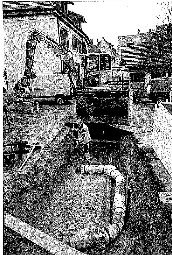
Fig. 5: Installation of an expansion bend in a PE-HD gas pipe, Meiergasse, distance to the well field approx. 80 m in northnortheast direction, March 2009 (Photo: U. Burbaum).
